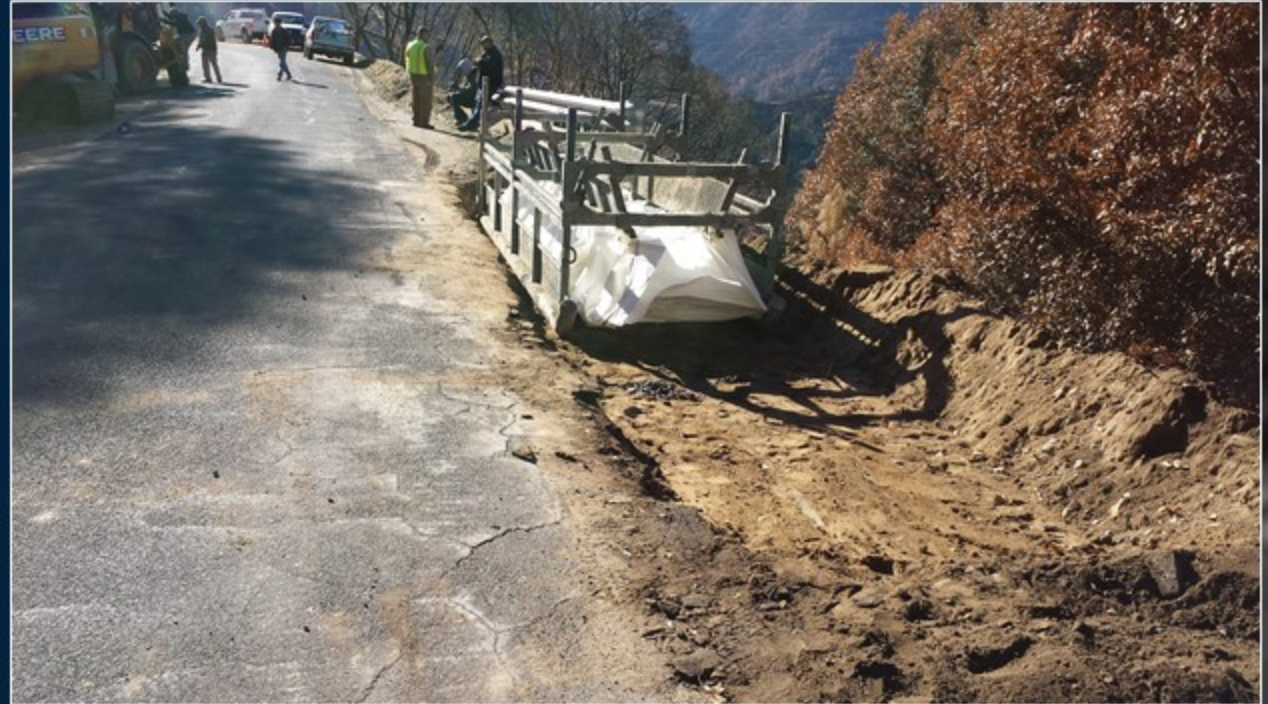
The PermaShield™ installation sled is set into place at edge of headwall
