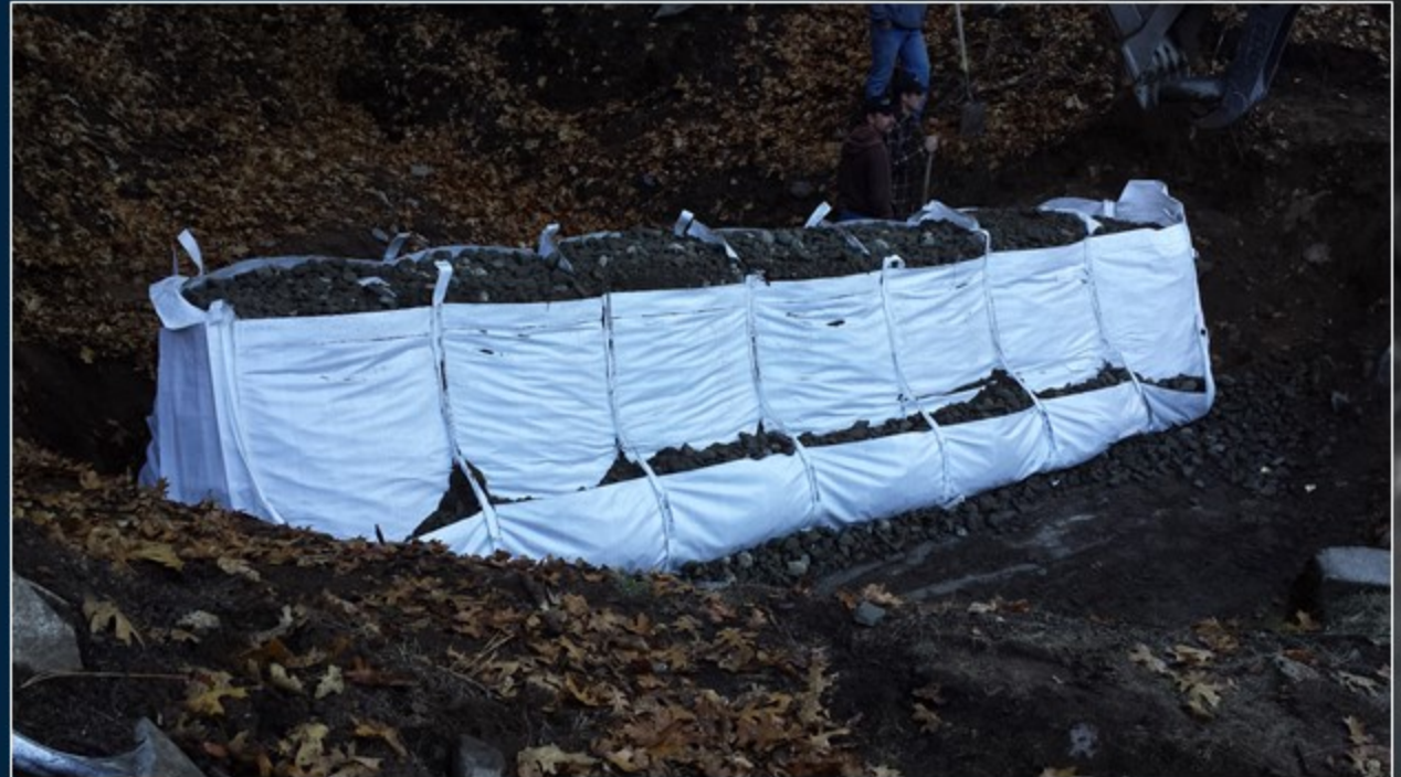
FlexiShield™ system installed and ready
