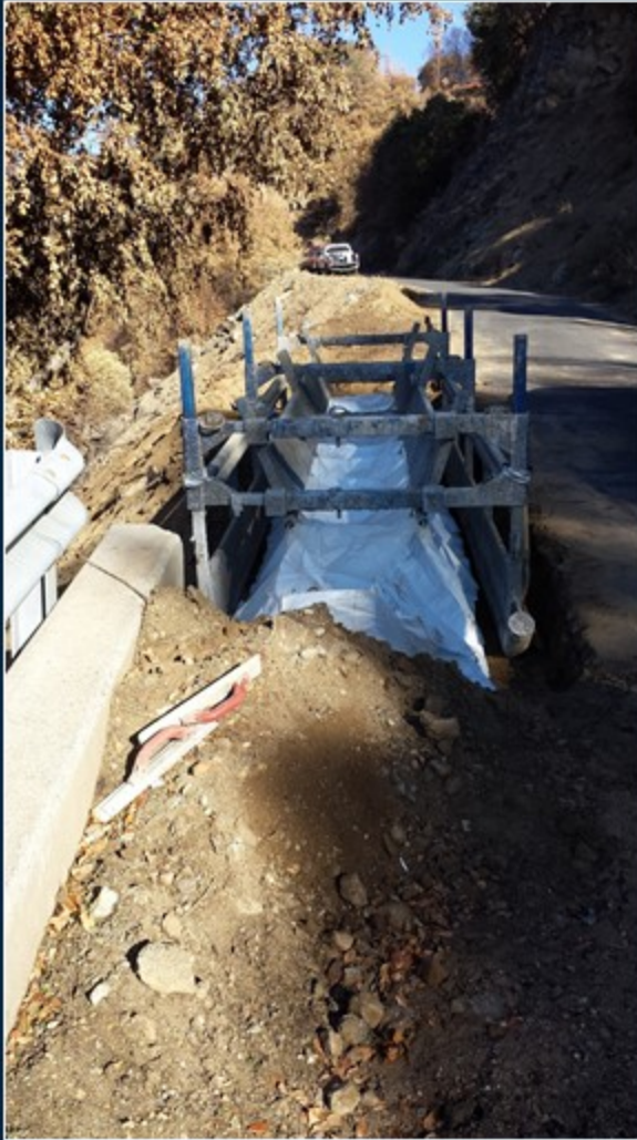
Looking uphill where rainwater generates velocity
