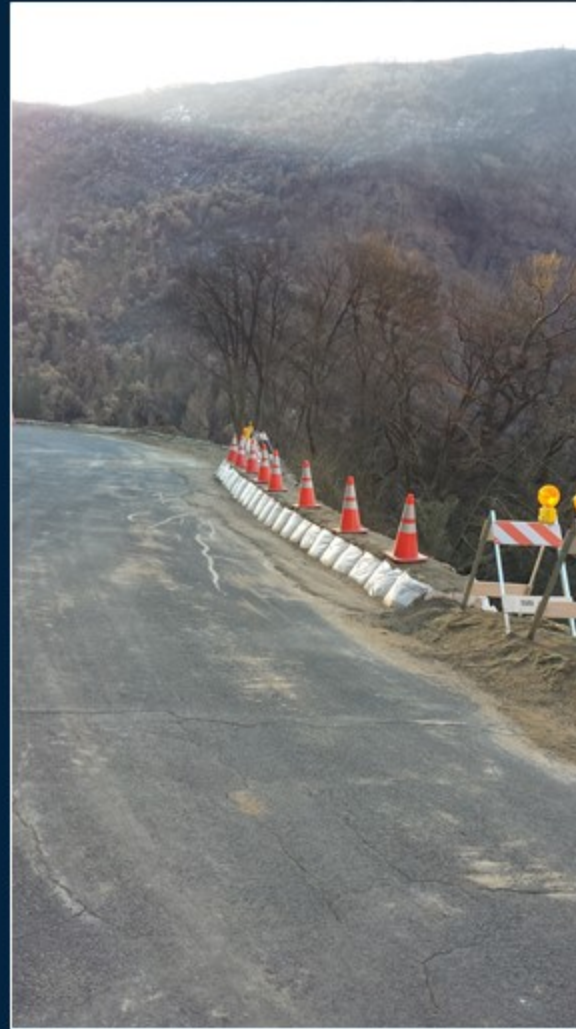
PermaShield™ buried 1' beneath surface
