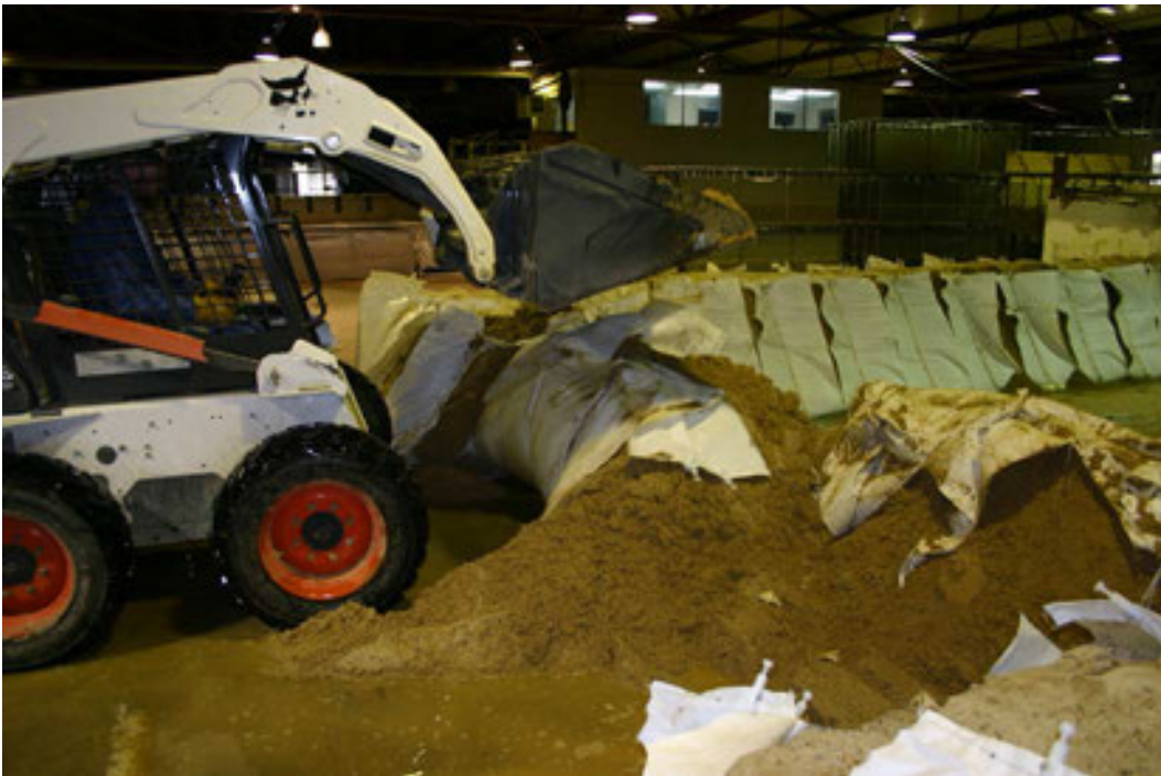
Figure 47. A skid-steer loader is used to roll the bags over, dumping out the sand.
