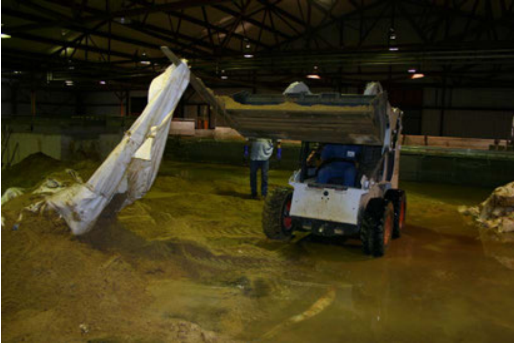
Figure 48. One extension fork is fastened to the front of the bucket to remove the bag material from the sand.
