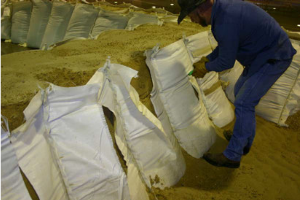
Figure 46. For removal, a box cutter is used to slice open the bags on both the inside and outside.
